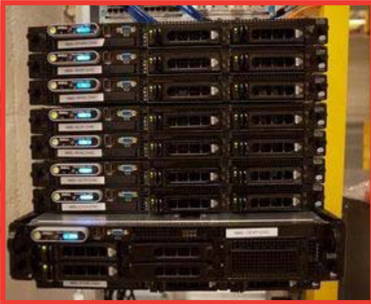
◀ Typical Internet2 Network point of presence (PoP) equipment setup.
